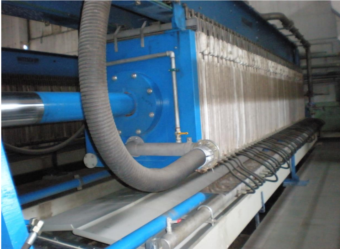
Fig. 3.15. General view of the filter press.
